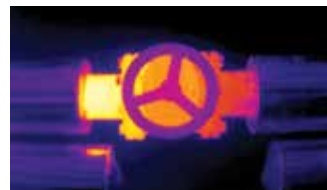
Thermal camera view of the uninsulated valve
